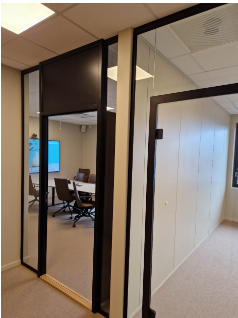
Figure 2. Flanking wall in corridor splitted.
