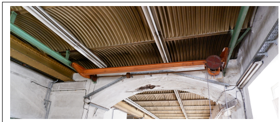
Figure 2. Existing industrial indoor crane used for mounting the sound absorption panel.
