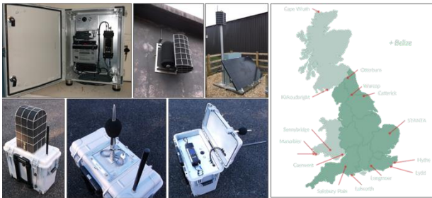
Figure 3 - Sample images of the current GNAT Noise Monitoring Systems showing permanent installation in the upper images and portable systems in the lower images. Both feature extensive wind noise rejection measures. The locations of the permanent systems are also indicated.
