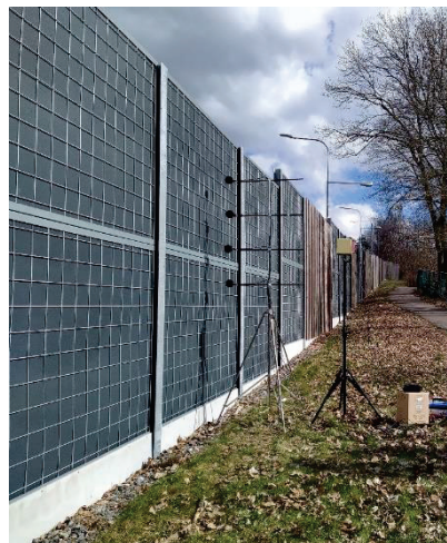
Figure 5. The measurement site of the Torpa school barrier. The school area is to the right in the picture.
