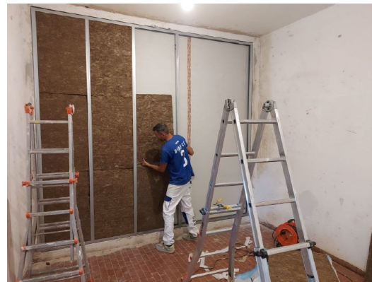
Figure 7. Installation of the self-supporting wall lining on the receiving room (internal side), insulated with 40 mm of rock wool
