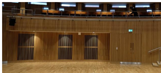
Figure 4. Side walls with air diffuser (darker areas).
