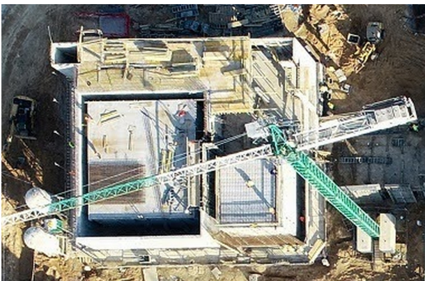
Figure 6. Acoustic lab without a roof, with box-in-box structure around both anechoic chambers clearly visible
