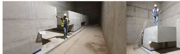
Figure 11. Author (for scale) next to 60tons floating foundation blocks, supported temporarily on 100mm thick elastomeric pads.
