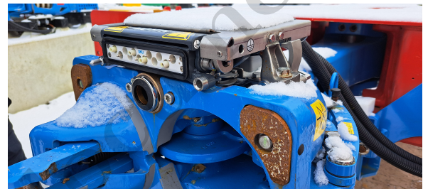
Figure 1: Couplings between train wagons include many different types of bolted connections which get loosened after continuous vibration.
