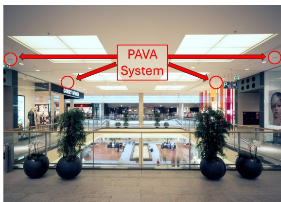
Figure 4. Public address voice alarm (PAVA) system installed in the ceiling of a shopping centre in Braunschweig, Germany.
