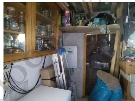
Figure 1. Solar inverter installed on the wall of a private garage.
