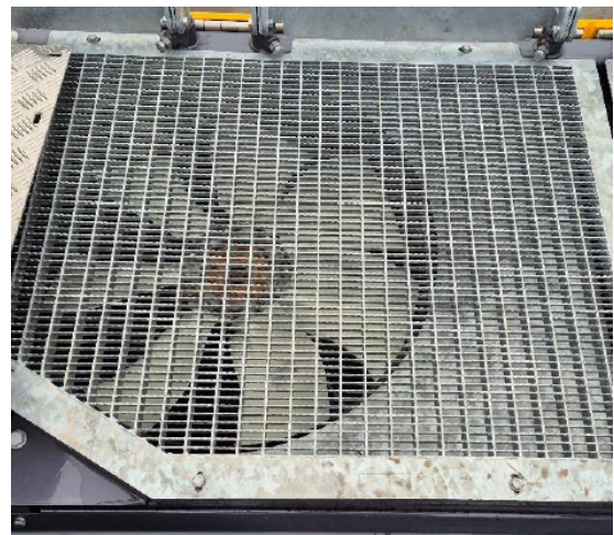
Figure 1: Example of an axial fan as part of a cooler-unit in a rotary drilling rig protected by a grille.
