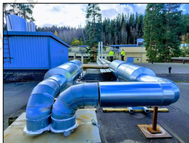
Figure 2. Two units of the three-unit silencer system visible in two adjacent exhaust ducts.
