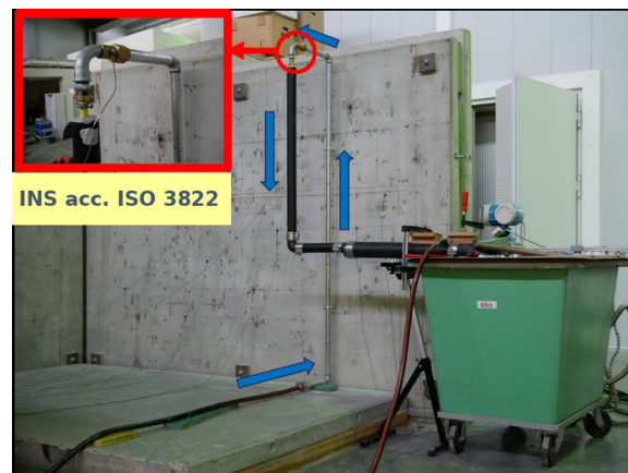
Figure 2 – Freshwater piping system mounted and operated on the reception plate test bench according to EN 15657. Blue arrows indicate the direction of the water flow.
